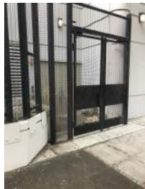
MAC service room door on Nagle Place
